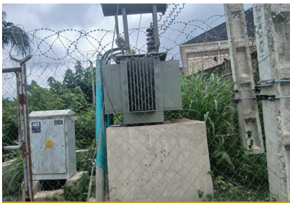
TRANSFORMER, AKURO PHASE 2
