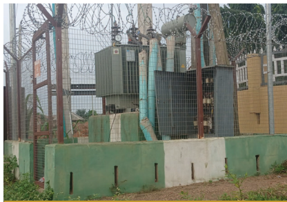
TRANSFORMER, OSILARU STREET
