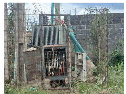
SWITCHGEAR AND FEEDER
