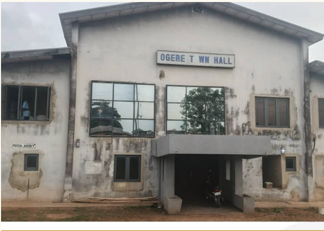
THE HALL TODAY — EXTERIOR AWAITING REHABILITATION
